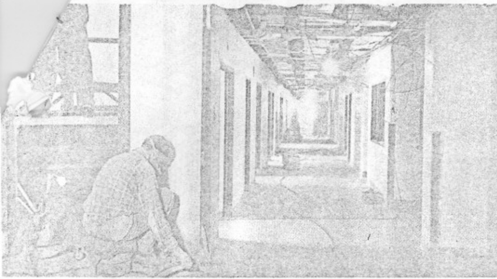
CURRENT PHASE OF EXPANSION is nearing completion and will be finished this winter. At left, workmen, windows and scaffolding create an interesting pattern as finishing touches are put to new patient rooms. Photo at right looks down a wire-strung corridor on the new seventh floor of the West Wing. Thirty-six patients will be housed in this area.
